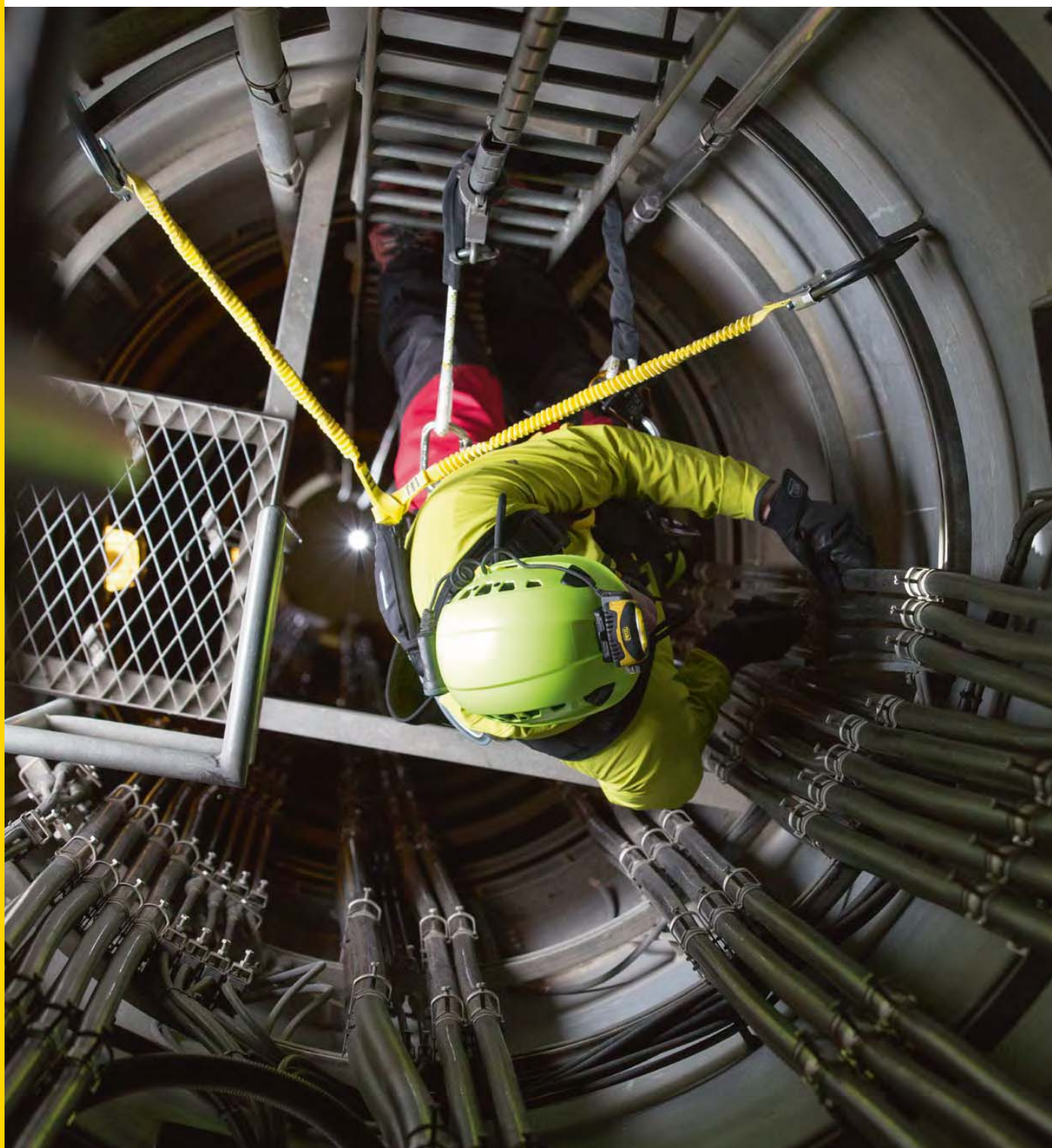
Maintenance work on the Monte San Salvatore tower in Lugano, Switzerland. © Petzl / Lafouche / Swisscom Broadcast / Etavis
